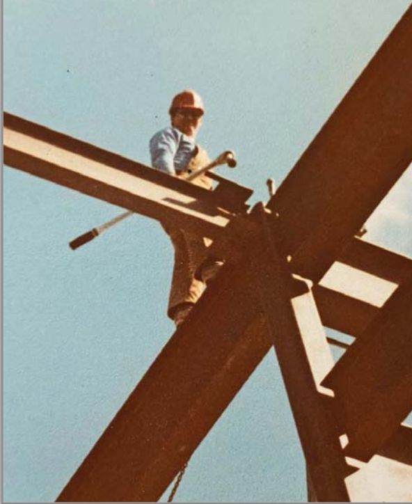
Ron Umlandt atop steel beams at the Fort Meade Commissary in Maryland in 1984, the year before he founded Tri-State Steel Erectors, Inc.
