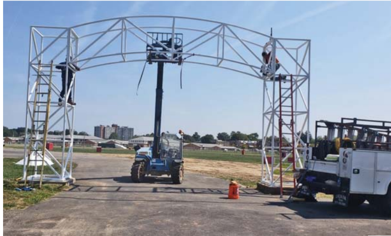
After an aluminum marquee at Baltimore’s Pimlico Race Course blew over, Tri-State Steel Erectors, Inc. replaced it with a white-coated steel structure.
