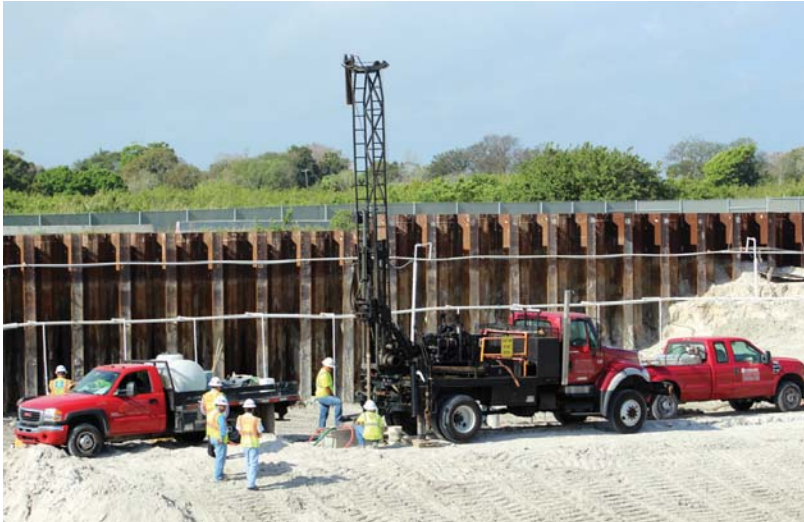
Universal Engineering Services, Inc. and GFA International, Inc. have both provided a range of services to the U.S. Army Corps of Engineers for rehabilitation of the 143-mile-long Herbert Hoover Dike in South Florida.
